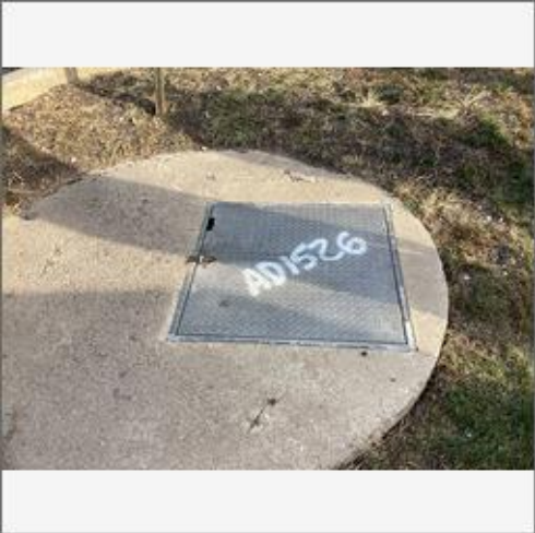
Valve Vault Access Hatch
