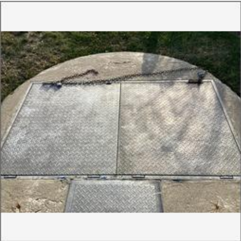
Wet Well Access Hatch
