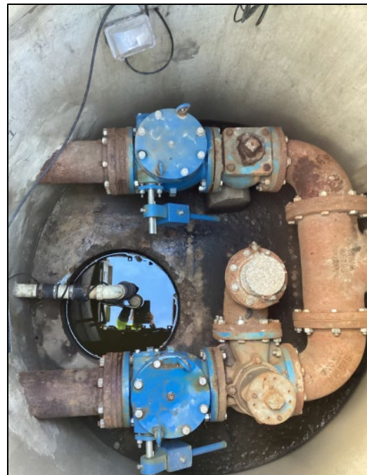
Figure 5 – Valve Vault Topside
