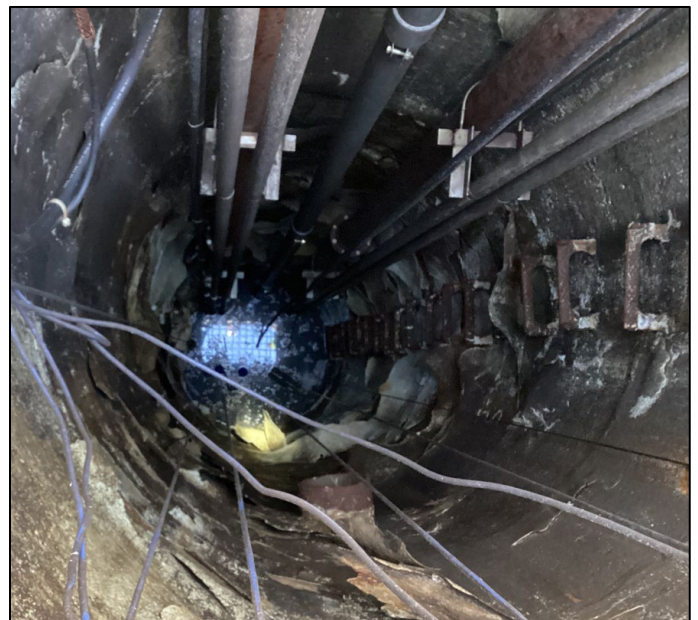
Figure 2 - Cementitious Liner Deterioration
