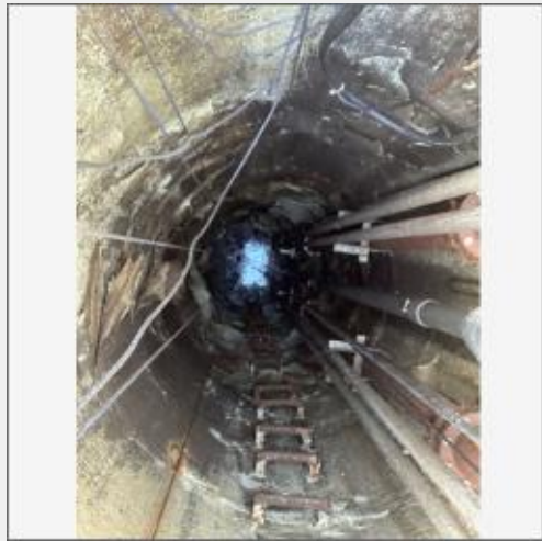
Wet Well Topside
