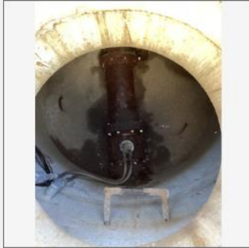
Flow Meter Vault
