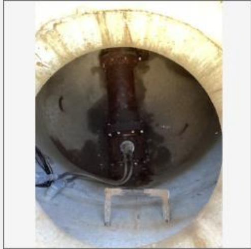
Flow Meter Vault
