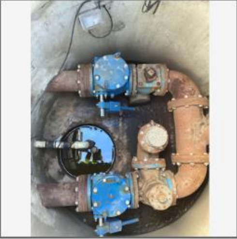
Valve Vault Topside
