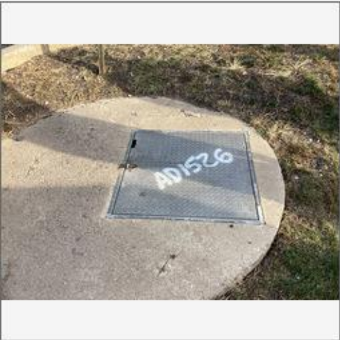
Valve Vault Access Hatch
