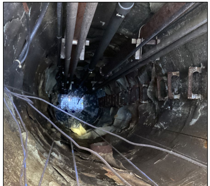
Figure 2 - Cementitious Liner Deterioration
