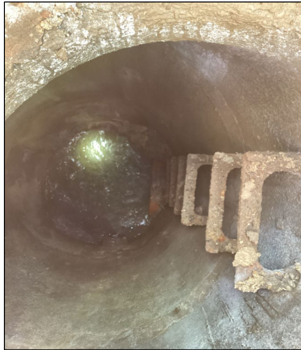
Figure 4 – Discharge Manhole Corrosion
