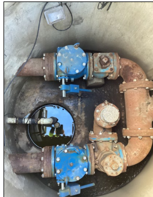
Figure 5 – Valve Vault Topside
