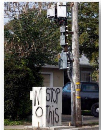
Recent Example of Poorly Managed Wireless Infrastructure Deployments
